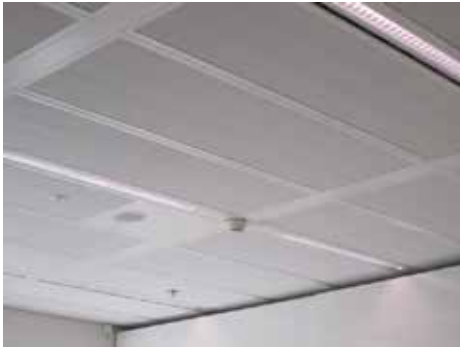
The passage of hot water can be clearly seen in the thermal image (right).
