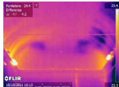
In this thermal image the dark spots indicate moisture ingress in the vaults of the Museum of the Academy.
