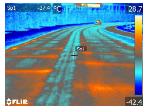
Thermal imaging can be used to see whether cooling devices of road infrastructures are working effectively.
