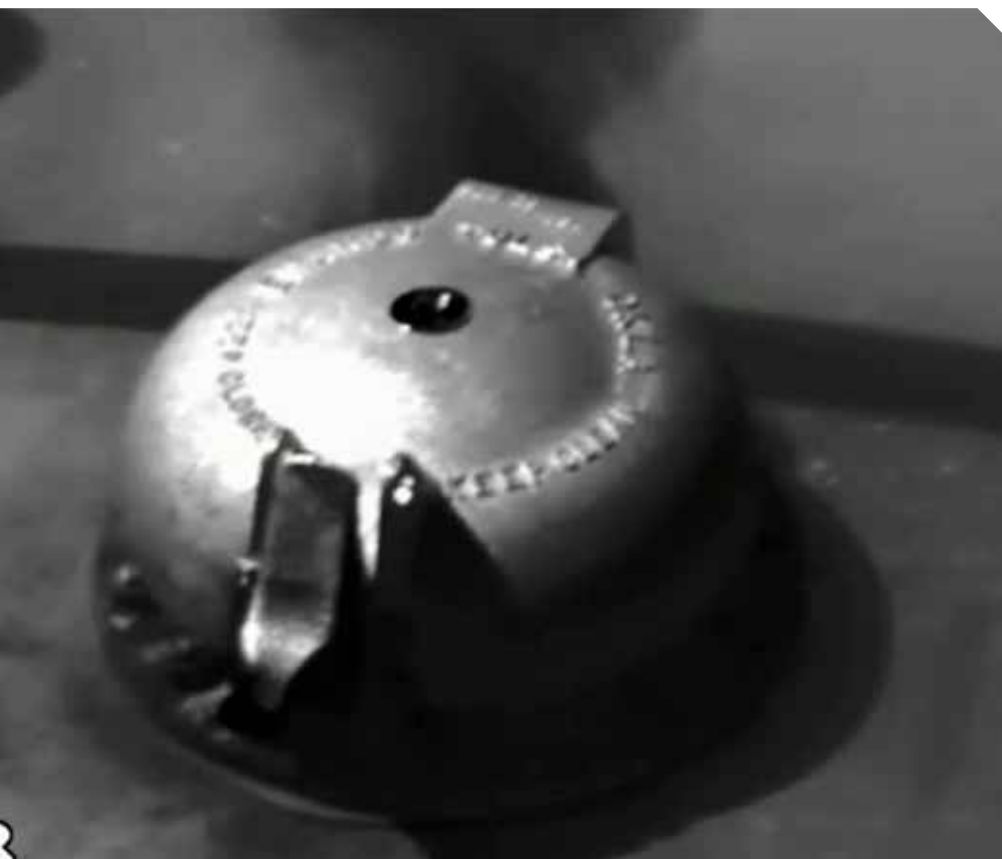
Optical gas camera shows methane leaking from thief hatch
