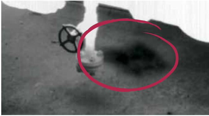
Captured gas leak from production site.
