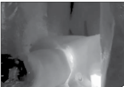
Leak in a 4-way valve dryer skid
