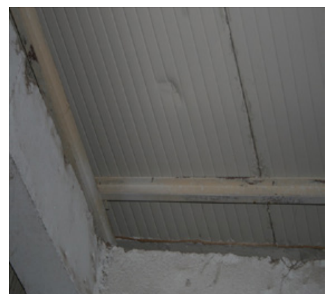
Leaks in the insulation material covering the cold storage unit can be a threat to the temperature uniformity inside the unit.
