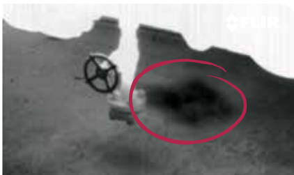
Captured gas leak from production site.
