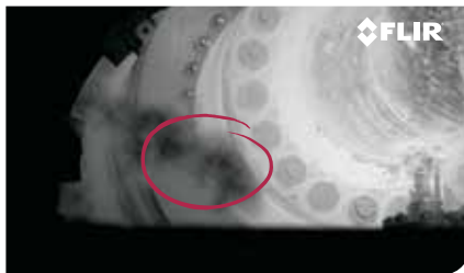
A leaking flange.
