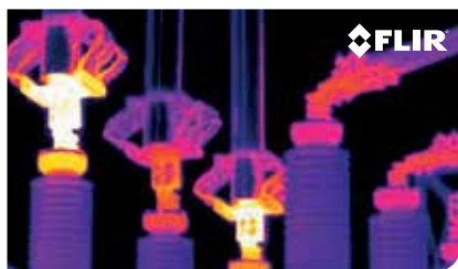
Thermal image of a substation showing a transformer with excessive temperature.
