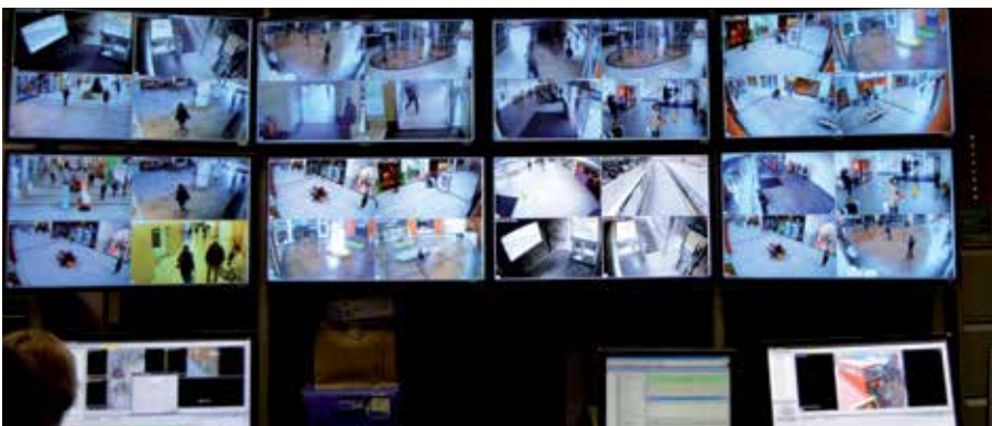
All camera video feeds are terminated within the Centre's control room, which is manned 24/7.
