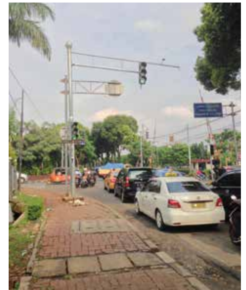
The ATCS system can be used to form a wave of green lights over several intersections.
